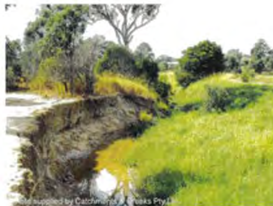
Photo 4 – Bank undercutting (Qld)
